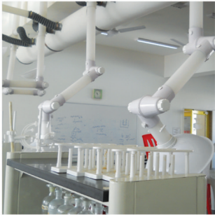
Ceiling Mounted Extractor
